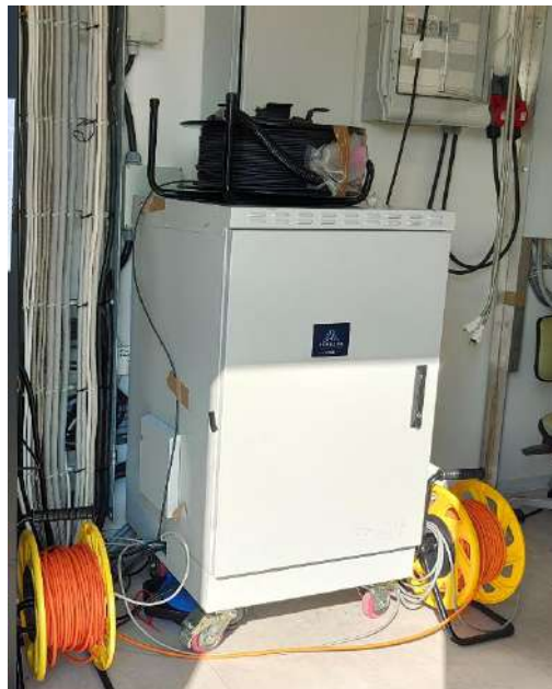
Figure 5 – Electrical support rack of SERA IV placed near of the launch rail inside an electrical container
